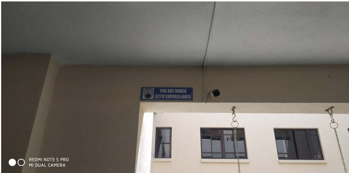
CLOSE CIRCUIT CCTV CAMERA AT ALL MAJOR POINTS
